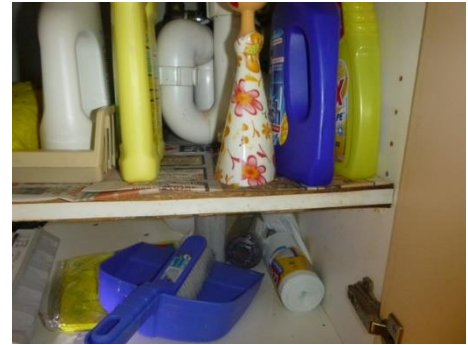
The cabinet and shelf of the kitchen sink cabinet has deteriorated due to moisture exposure
