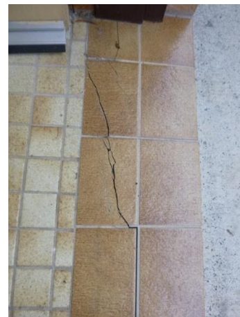
Cracked threshold tiles
