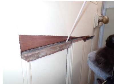
The northern external door is damaged at the base
