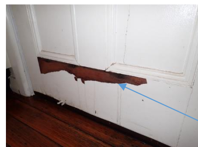
The eastern entrance door is damaged at the base
