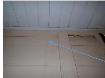
Drip marks present to the southern wall lining indicative of leakage from the valley gutter above
